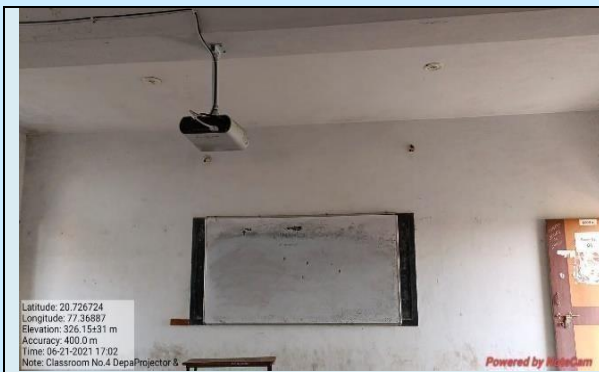
Classroom No. 4 With LAN & PROJECTOR
